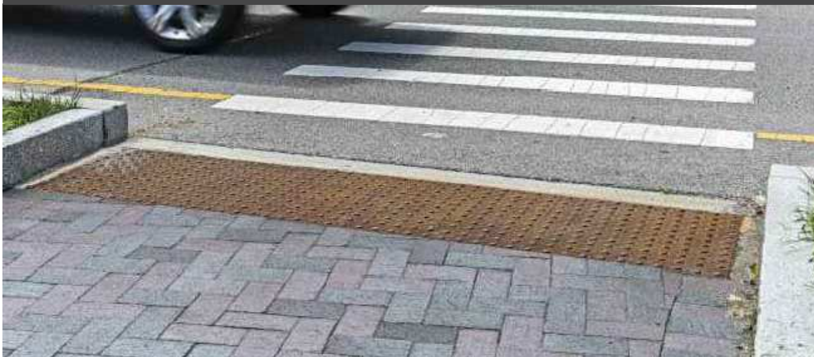
CAST IRON ADA TACTILE STRIP
