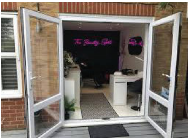
Garage conversion: Swapping the overhead garage door for french doors created space for a home-based salon business.
